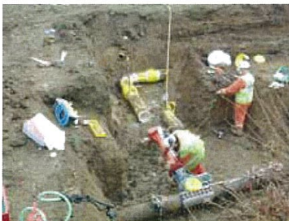
The type of environment where testing of pipe welds need to be conducted.
